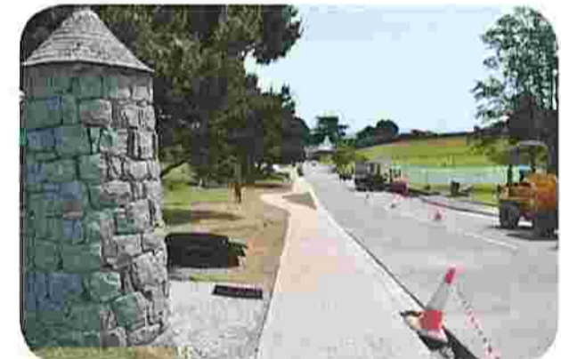
Above - The new meandering footpaths under construction, entrance walling and new planting beds.
