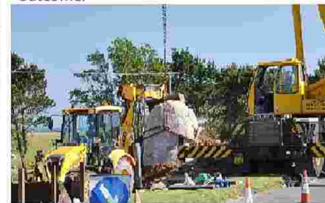
Above - The thirteen tonne boulder being craned into position at the Warren entrance to create a new feature sign.
